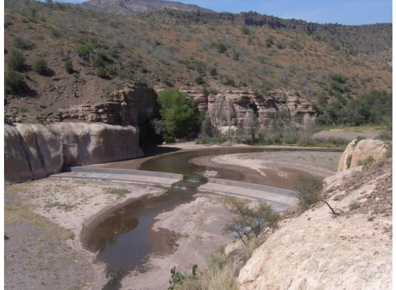
Figure 2. Completed Blue River fish barrier. Photo courtesy of Rob Clarkson, Bureau of Reclamation.
