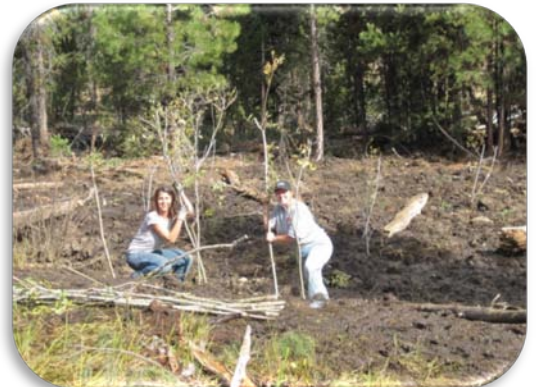
Figure 2. Paulina Botanist, Krista Lopez, and Anne Roberts planting willows, cottonwoods, and alder on a stream head cut repair project.
