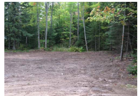
Figure 3. Cleared and shaped basin for rain garden at Forest Visitor Center/ District Office Complex
