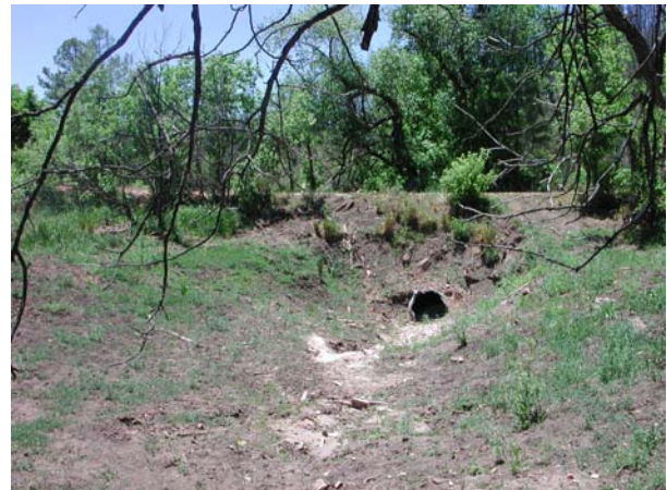
Figure 5: This road crossing at Swamp Spring likely contributed to the extensive downcutting of the meadow by concentrating flows and failing to pass sediments and debris.
