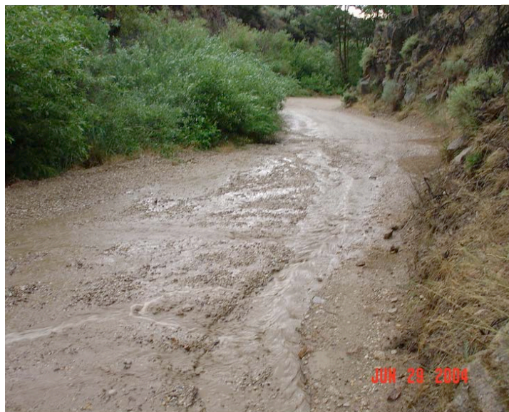
Roads create low-infiltration strips in a high-infiltration environment (for example, the surrounding forest in this photo) and are a major cause of erosion in forests. Here, the road is showing erosion due to poor surface drainage (photos from http://www.fs.fed.us/GRAIP/gallery/ ).
