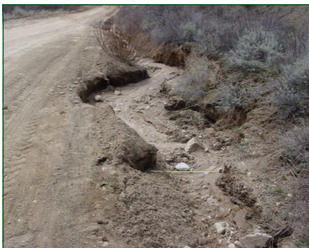
Road erosion and runoff produces fine sediment, contributing to increased sediment yields.
