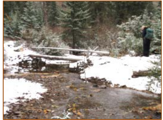
An old ford stock crossing Holland Creek (foreground of photo) in shallow water and gravel bar was stabilized, and the log foot-bridge was replaced in FY15.
