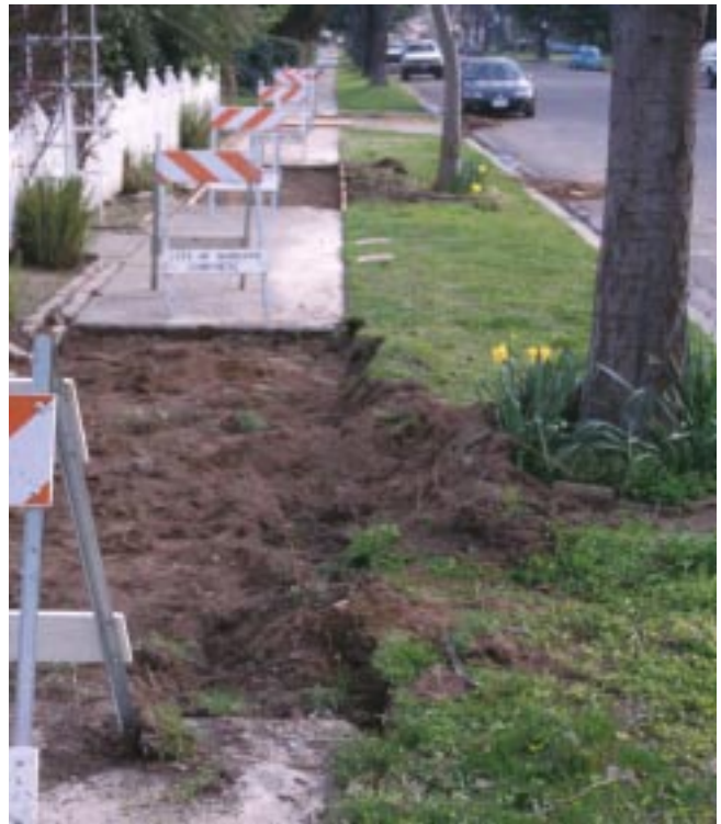
Figure 1. Sidewalk damage caused by tree roots is commonly found in California. Annual repair costs are substantial.
