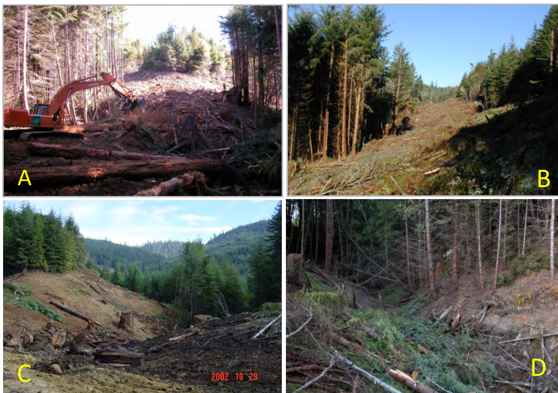
Figure 2—A. stream crossing being excavated; B. outsloped road with heavy mulching; C. recently excavated stream crossing with large woody debris placed within the exhumed channel; D. excavated stream crossing with a relatively large volume of woody debris added.
