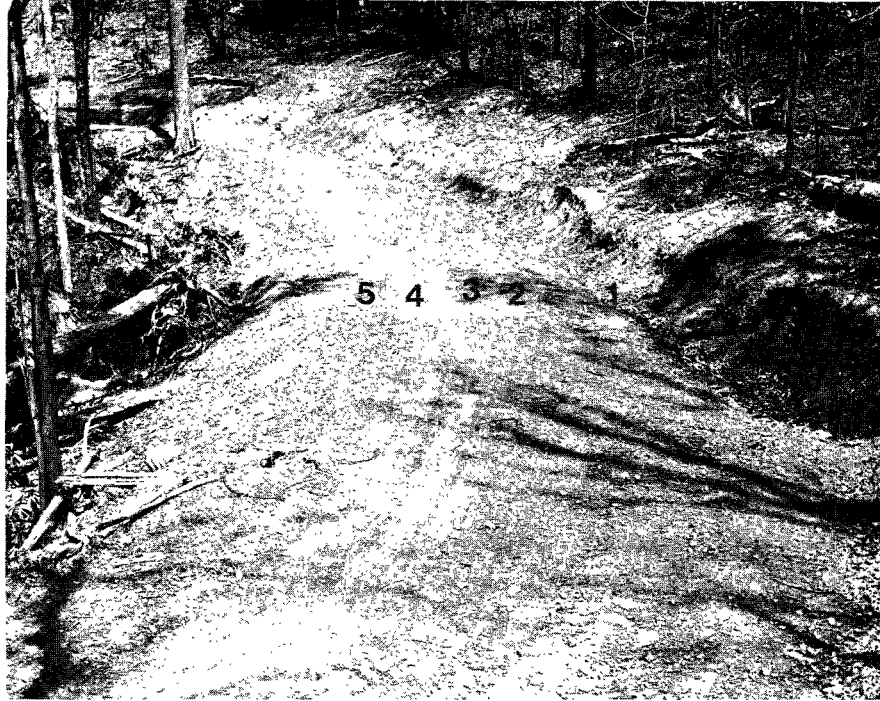
Figure 2.—A minimum-standard road section with a high percentage of coarse fragments. Note the density sampling sites in the upper half of the photograph. The numbers refer to the measurement points on a transect.
