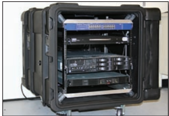
Figure 1— A terminal server is the heart of the thin client kit. The server and other hardware are mounted in a rugged case for protection. It will be transported and operated inside an air-conditioned trailer at the incident.
