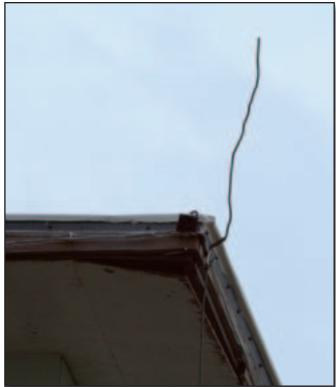
Figure 1a—This improper substitute for an air terminal is made from copper wire.
