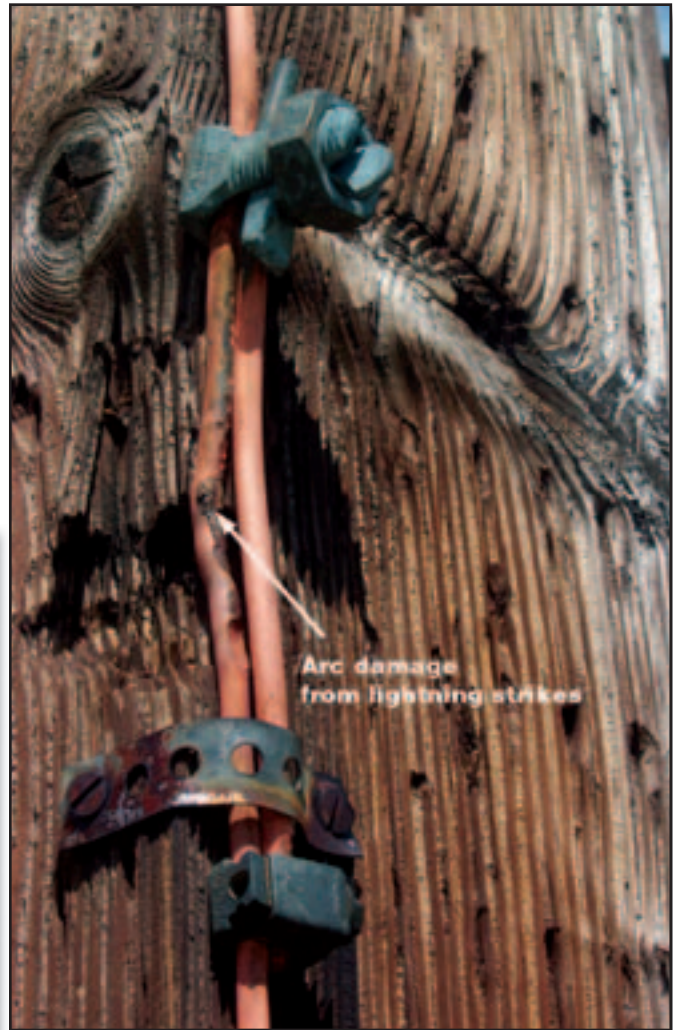
Figure 3—This wire junction doesn’t use connectors approved for lightning protection on down conductors. Note the arc damage from lightning strikes.
