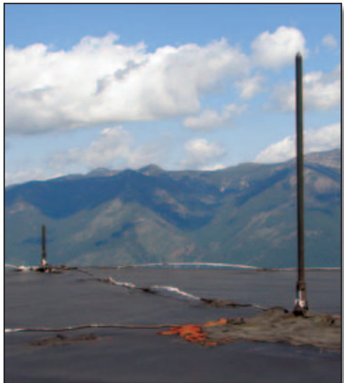
Figure 1b—These proper air terminals are constructed of ½-inch diameter copper rods and have at least two conduction paths to an earth ground.
