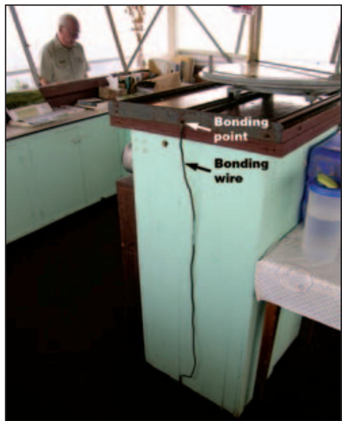
Figure 4—This bonding wire is attached to a fire finder inside a Forest Service lookout.
