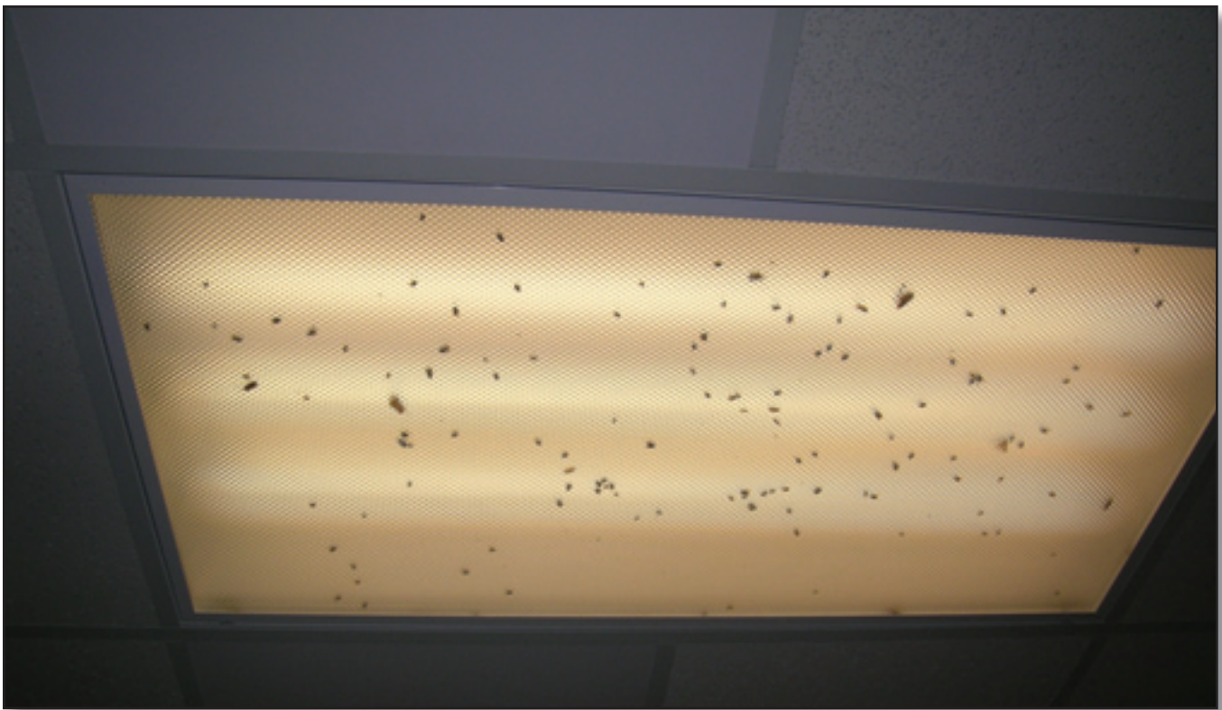
Figure 5—A fluorescent lamp with a luminaire that needs to be cleaned or replaced.
