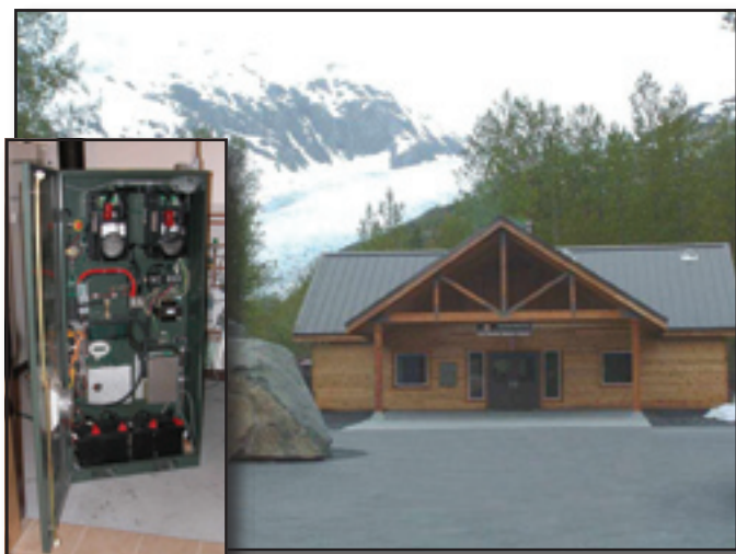
Figure 3—This fuel cell (inset), similar to the model used at Big Goose, provides electricity reliably for the Exit Glacier Nature Center at Kenai Fjords National Park in Alaska.
