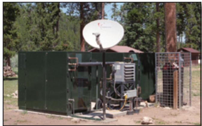
Figure 1—Two 5-kilowatt fuel cells were installed at Big Goose Ranger Station during the summer of 2005.
