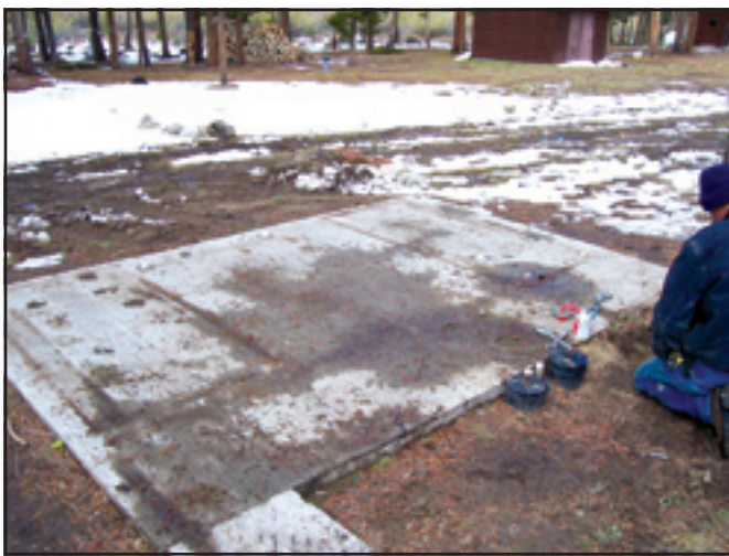
Figure 2—The fuel cells were removed from Big Goose Ranger Station in September of 2006.
