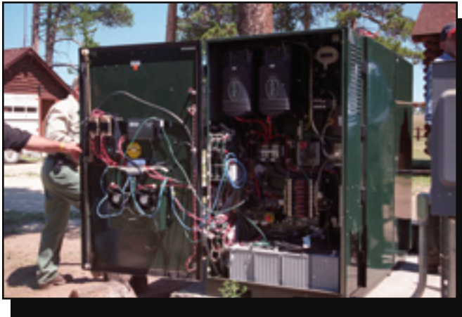
Figure 4—The Acumentrics Corp. provided information to Forest Service personnel so they would understand the basics of the components in the fuel cells and their operation.
