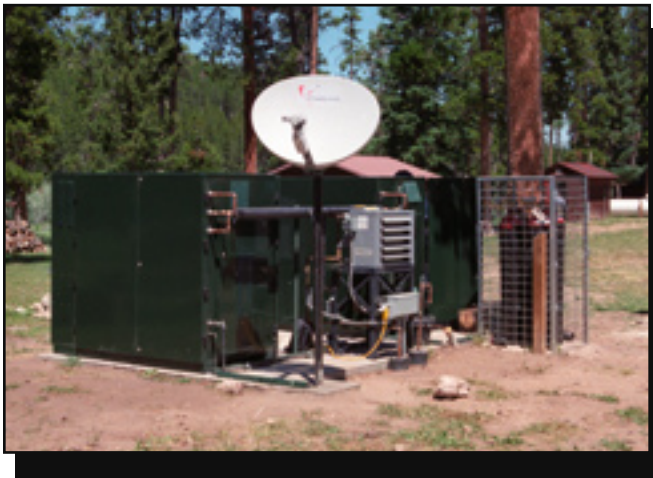
Figure 1—The completed fuel cell installation at Big Goose Ranger Station in Wyoming.
