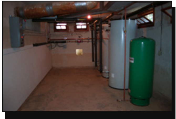
Figure 3—The hot water storage and expansion tanks are in the basement of one of the bunkhouse cabins.
