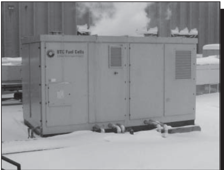
Figure 4—Steam vents from the top of a 200-kilowatt, model PC 25 fuel cell manufactured by UTC Fuel Cells. The unit can produce uninterrupted power for critical needs such as hospital life support equipment, computer centers, or emergency services, in addition to providing electrical power for more ordinary uses. —Photo courtesy of Concurrent Technologies Corp., Johnstown, PA.
