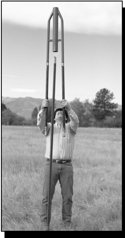
Figure 7—The driver is being lifted off the top of a post after the Standard-Signs NO4 post has been set.
