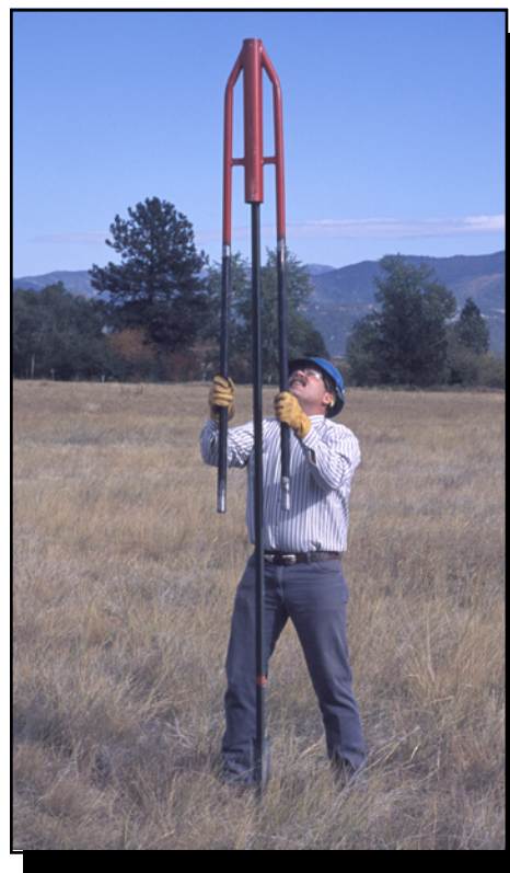
Figure 6—Driving a 10-foot T-post into the ground with the Standard-Signs NO4 driver.
