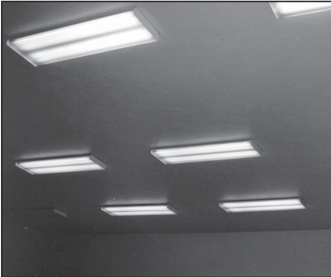
Figure 2—Typical 4-foot fluorescent lamp fixtures.
