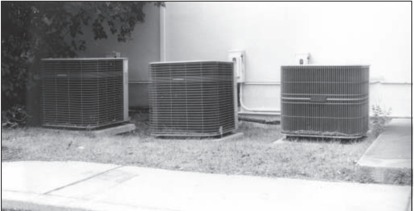
Figure 7—Three of MTDC's six air-conditioning compressors. Installing a controller that would prevent all the compressors from operating at the same time would lower MTDC's peak electrical demand.
