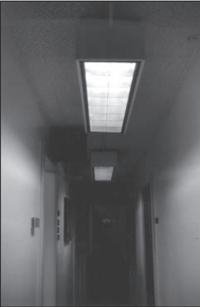
Figure 4—Light fixtures with energy-efficient T8 fluorescent lamps and electronic ballasts save energy and reduce peak demand.
