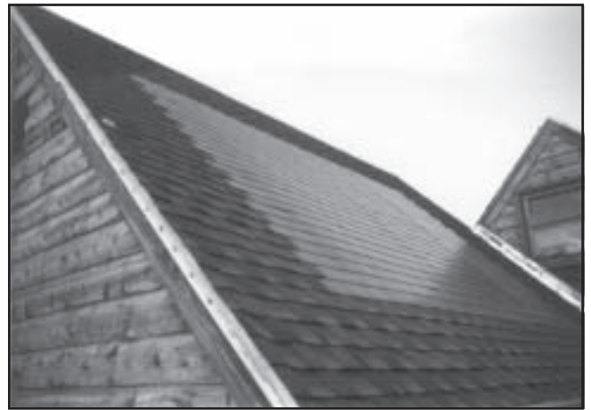
Figure 9—Photovoltaic cells on the roof of a Forest Service building. Photovoltaic cells produce power during the daytime when the peak demand for electricity usually occurs.
