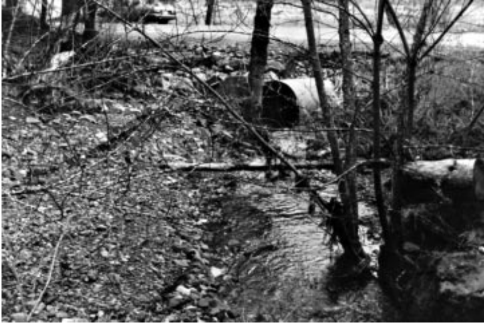
Figure 1—When compared with the bed width, the zone of average annual bedload transport, this culvert is undersized. Hydraulic calculations show this pipe unable to pass a 10-year design discharge. Also note terrace development. Such physical features often coexist and provide evidence for inadequately sized culverts.
