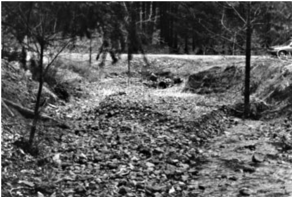
Figure 3—Terraces upstream of the culvert inlet indicate past ponded conditions. Channel dimensions and hydraulic capacity of this culvert should be checked.
