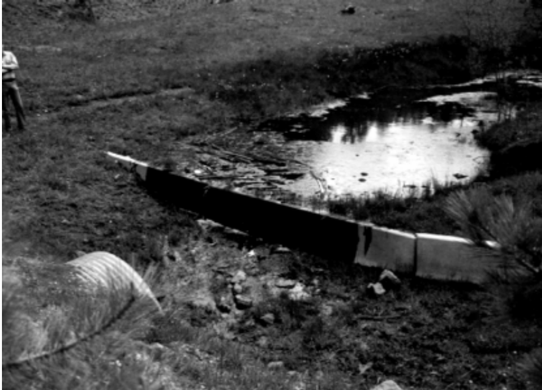
Figure 3—Jersey barrier gully plug.
