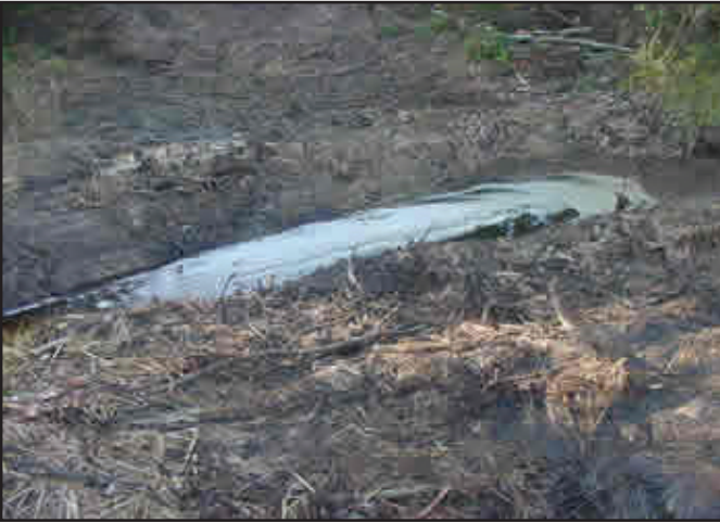
Figure 4—A closeup of the channel after removal of the temporary crossing. Note the indentations of the logs.
