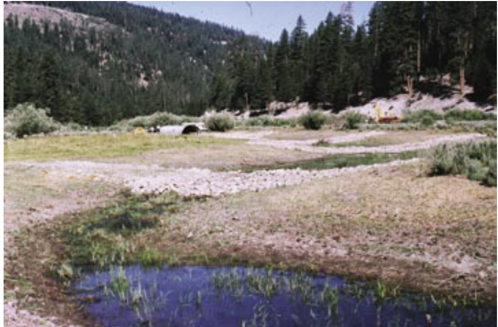
Figure A55. Looking upstream at the rehabilitated channel during placement of the culvert in 1988.
