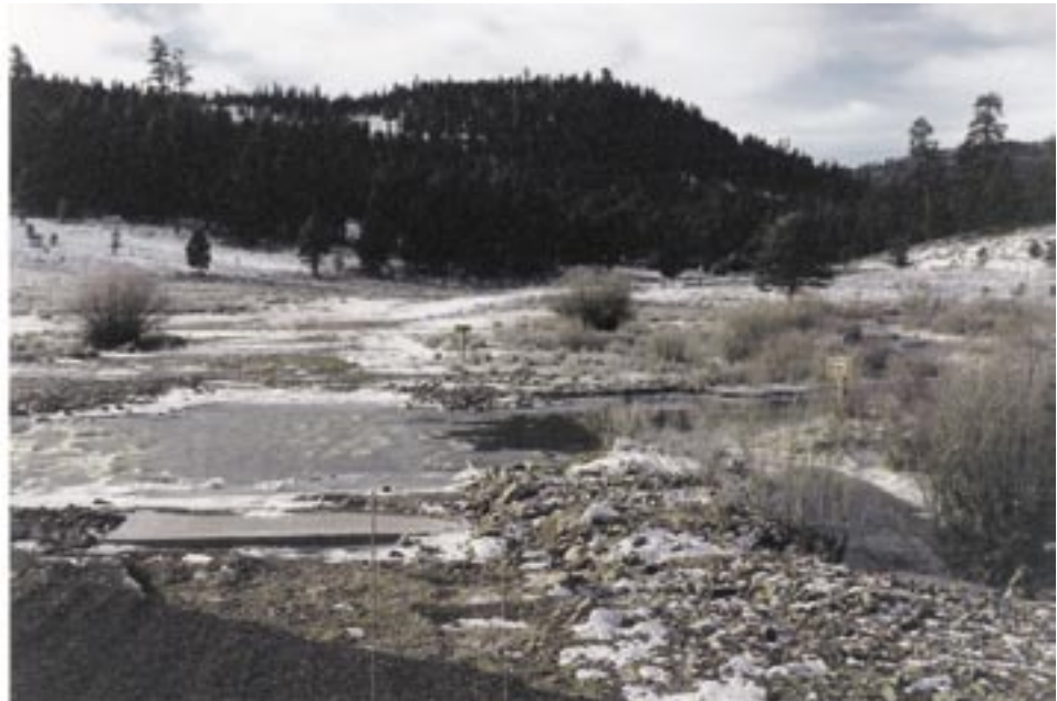
Figure A59. Shortly after the 1997 New Year's Day flood. Some gravel washed from the approaches (in foreground) was the only damage from the largest flood on record.
