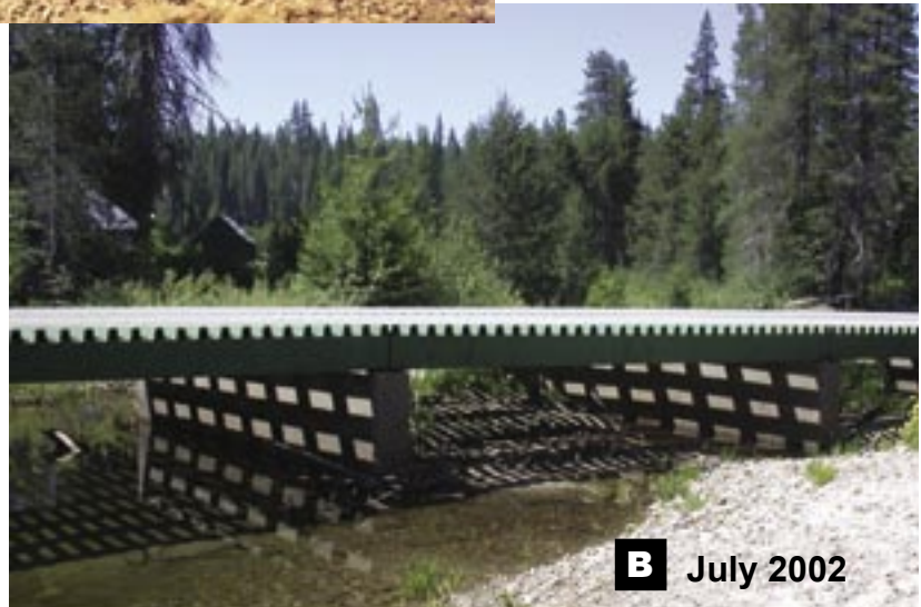
Figures A138a and A138b. Looking downstream at the Jones Wreckum Bridge. A138a. Bridge inspection photo.
