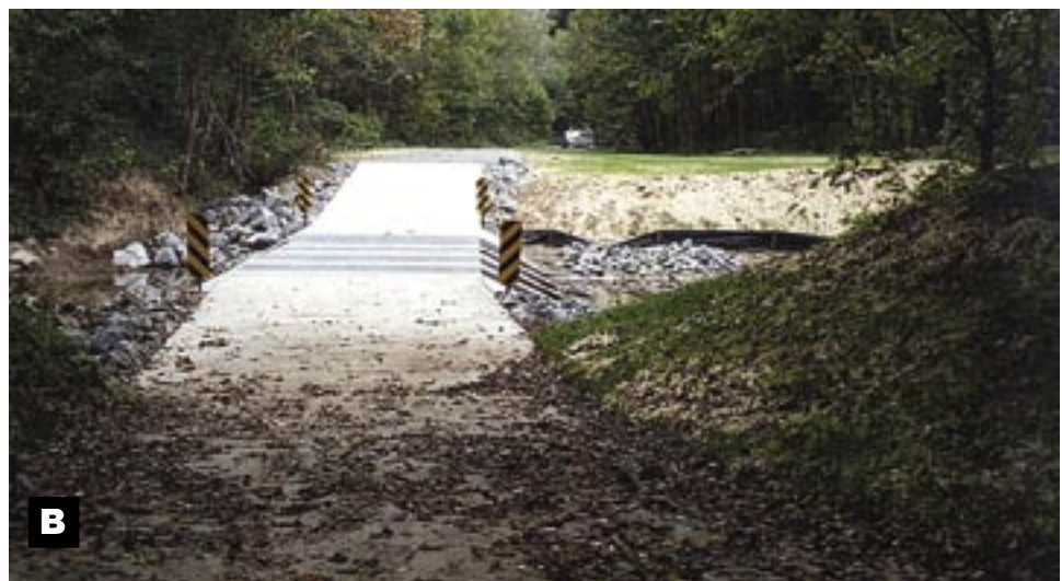
Figures A126a and A126b. Kinkaid crossing just after construction in 2001. A126a. Close up of embedded boxes; A126b. View along vented ford showing riprap.
