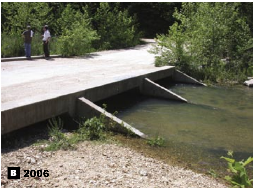
Figures A124a and A124b. Downstream side of the box culvert crossing. Between 2003 and 2006, gravel bar enlarged to block one box.
