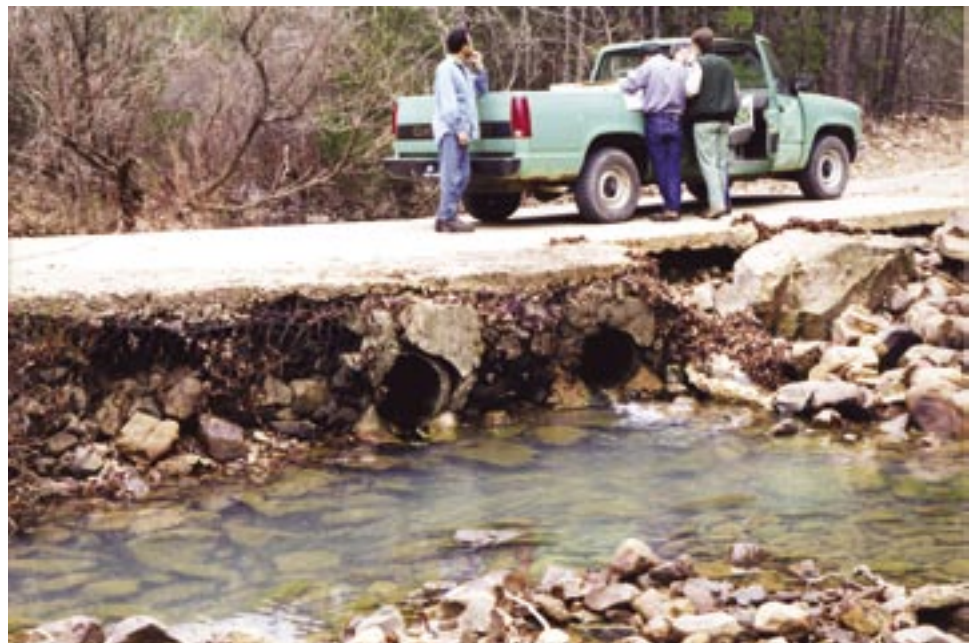
Figure A87. The previous crossing on road 887 at Rocky Creek was a gabion-culvert structure that was frequently damaged during high flows.
