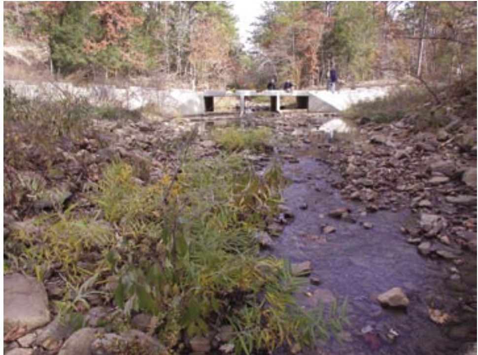
Figure A86. Looking upstream at the concrete vented ford and splash apron.
