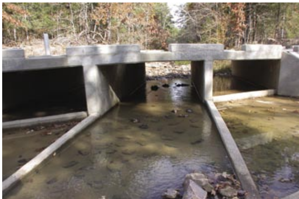
Figure A92. The floor of the central box has a thin veneer of sediment at low flow.
