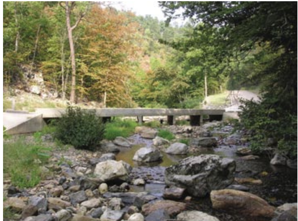
Figure A94. Looking upstream at the embedded box culverts that replaced the unvented ford in 2004.
