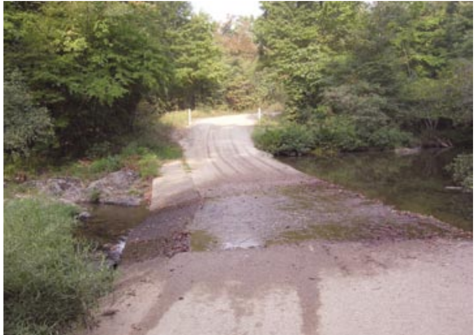
Figure A93. Unvented ford similar to the one replaced at FR 512 crossing on Long Creek, Ouachita National Forest.
