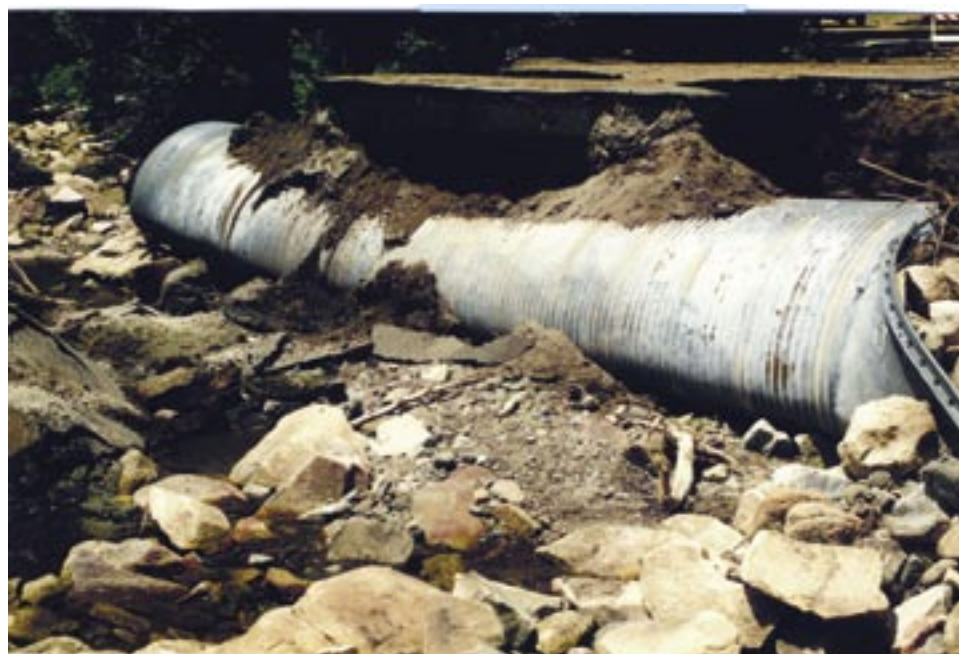
Figure A81. Typical flood damage at edge of North Fork Consumnes River valley after 1997 rain-on-snow flood.
