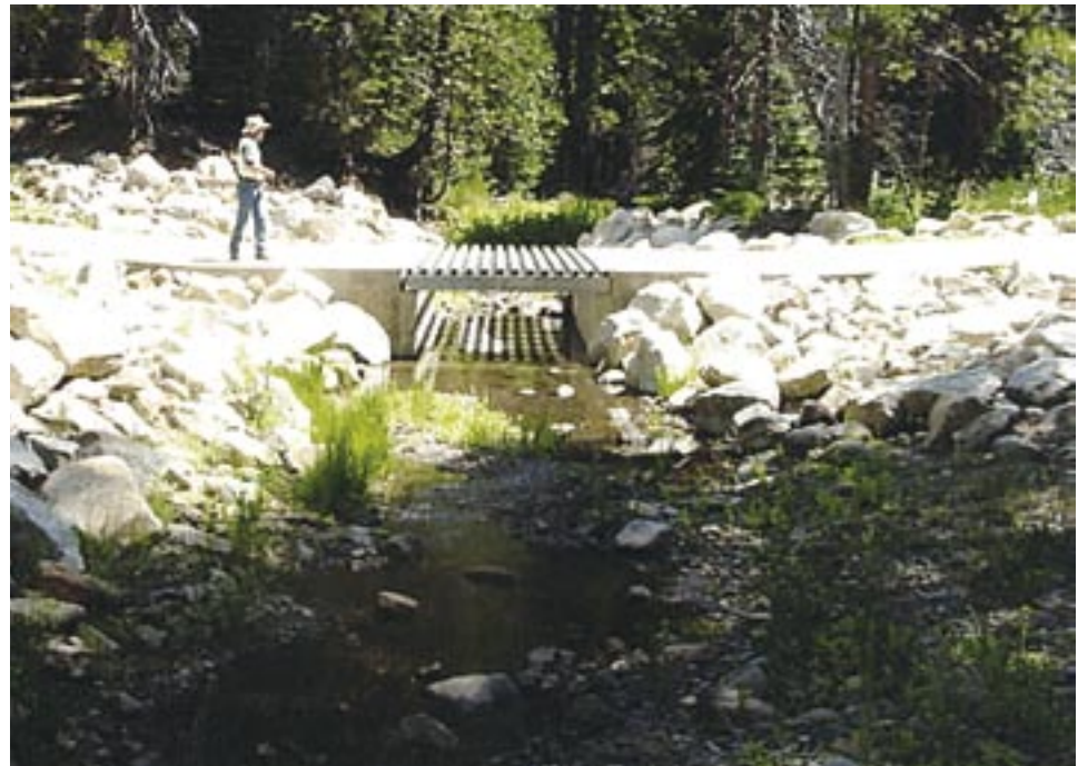
Figure A80. One of several grating-top box culvert fords on tributaries of the North Fork Consumnes River.
