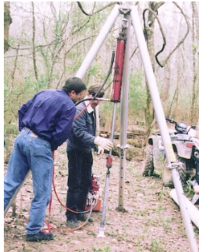
Figure 11—Once the probe is frozen a hydraulic cylinder is attached to hoist probe out of the ground.
