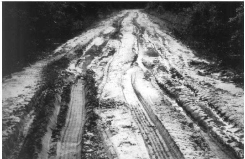
Figure 1. Rut development on Florida low volume road.
