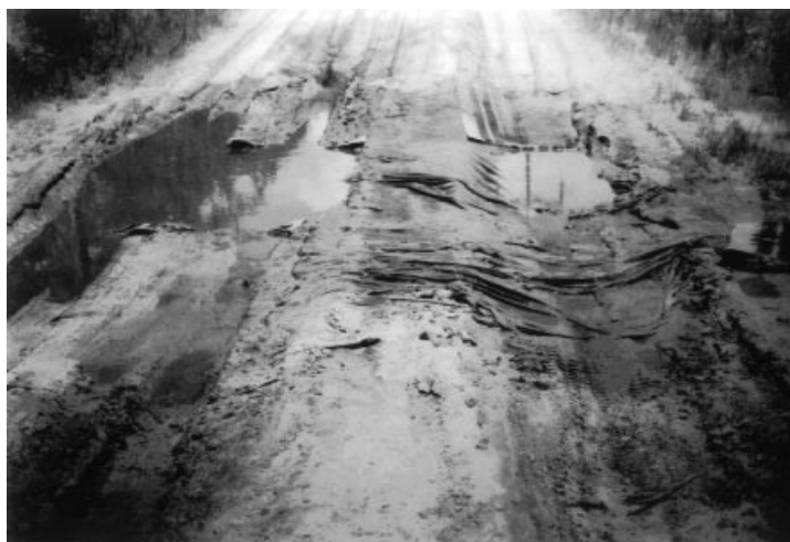
Figure 4. Portable surface and control sections, end of evaluation—Site 2.
