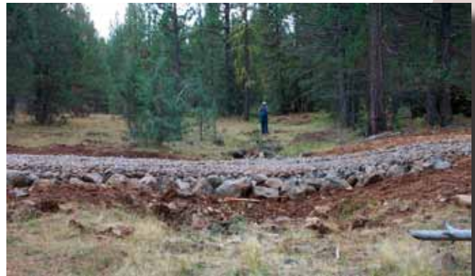
Armored dip on ephemeral stream in Lassen NF, immediately after construction in 2003. Photo by Carolyn Napper.
