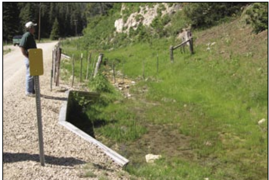
Figure 5—Culvert entrance as of June 2005. Note that the Sacramento Mountain thistle ( Cirsium vinaceum ) is beginning to grow in the entrance. We replaced and maintained fencing to keep cattle and other animals out of the thistle population. Photo: Nancy Taylor, Lincoln NF, R3.
