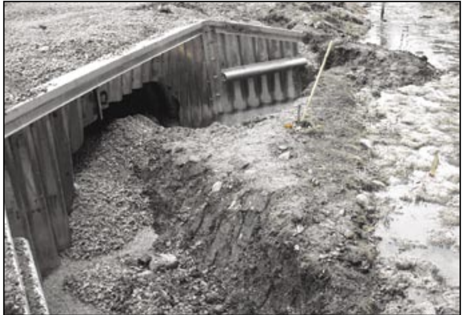
Figure 4—Aluminum pipe arch inlet during construction. Note that springwater is still diverted down the ditch to minimize flow through disturbed area. We did not allow the contractor to divert water with equipment. USDA Forest Service personnel diverted the water by hand by to minimize disturbance to the habitat. Photo: Tom Torres, Lake Tahoe Basin Management Unit, R5.
