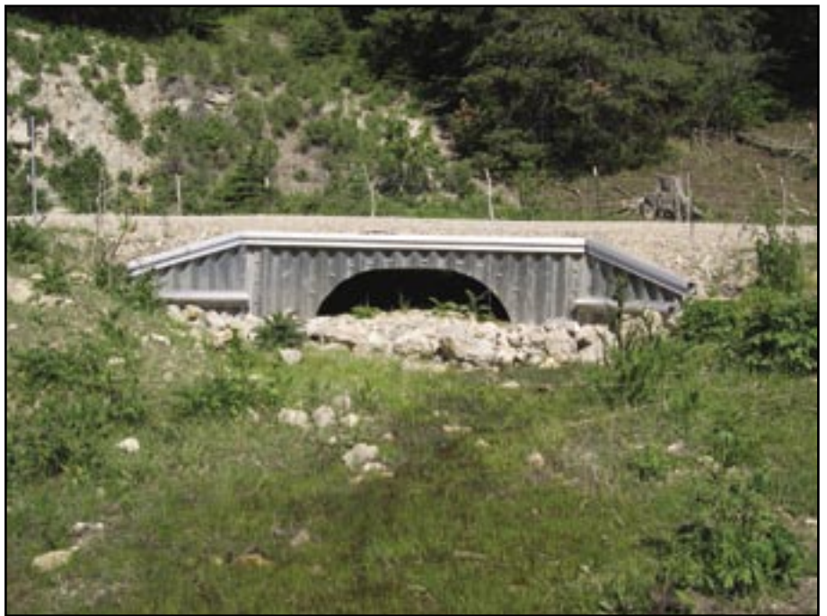
Figure 6—Aluminum pipe arch outlet. Photo taken June 2005. Note large arch opening requires only infrequent maintenance despite relatively large springflows. We constructed the road prism of 2- to 3-foot-deep permeable rock fill. The listed plant, Sacramento Mountain thistle ( Cirsium vinaceum ) is in the outlet of the structure.
