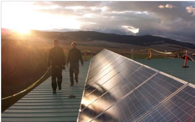
Twenty-panel 4 kW grid-tied system at the Pintler Ranger Station in Phillipsburg, MT, installed in 2009. This system is expected to produce a total of 5,500 kWh and prevent the release of 5,000 lbs of greenhouse gas into the atmosphere annually.
