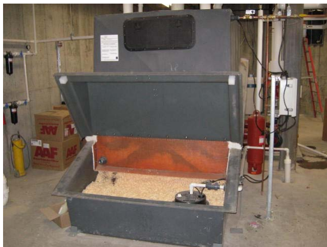
One of two composting toilet systems installed by Clivus New England, Inc., at the new White Mountain National Forest Headquarters, saving an estimated 70,000 gallons of fresh water annually, producing no methane GHGs, and ultimately making fertilizer. (Photo by Bill Dauer)
