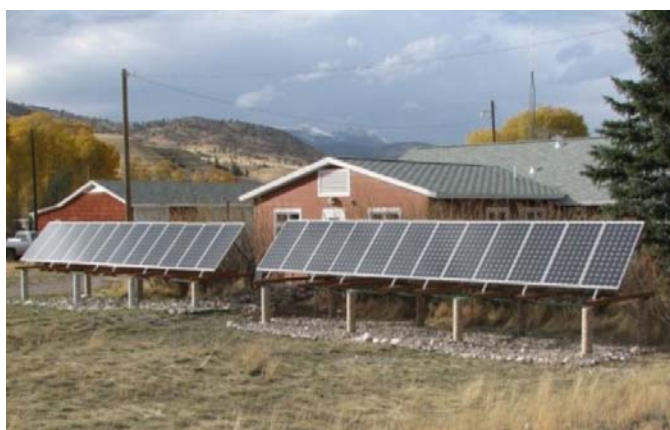
These solar panels were installed recently at a Madison Ranger District facility on Beaverhead-Deerlodge NF.
