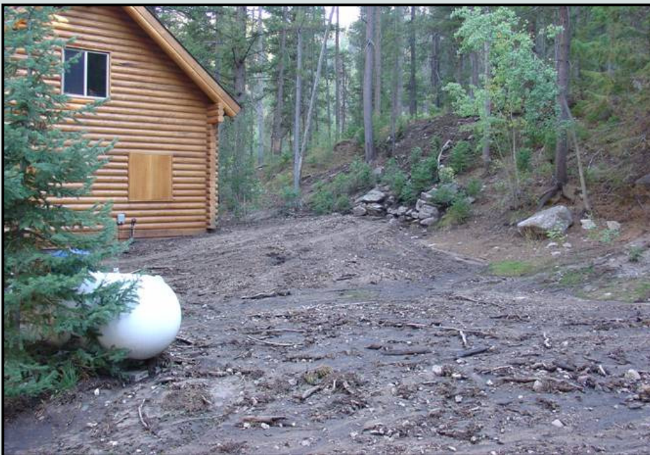
Even minor debris flows and landslides can have consequences in the wildland-urban interface.
