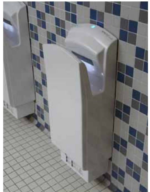
New efficient hand dryers recently installed in the visitor center restrooms
