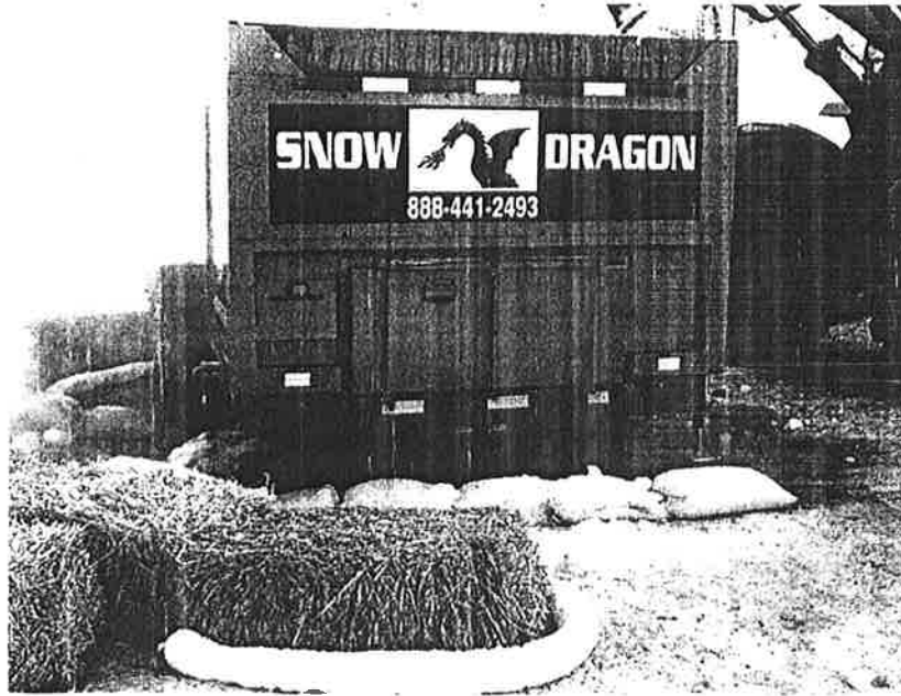
Photo 3: SND 900 in operation.
