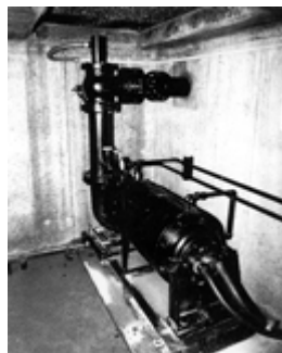
Self-Priming Centrifugal Pump with submersible motor in underground pit
