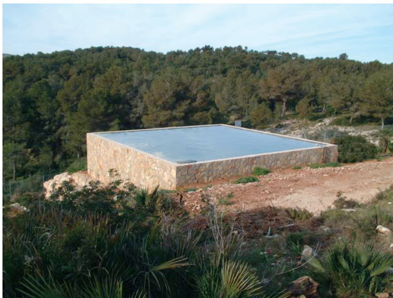
Figure 2 —Example of a water deposit for fire extinguishing services
