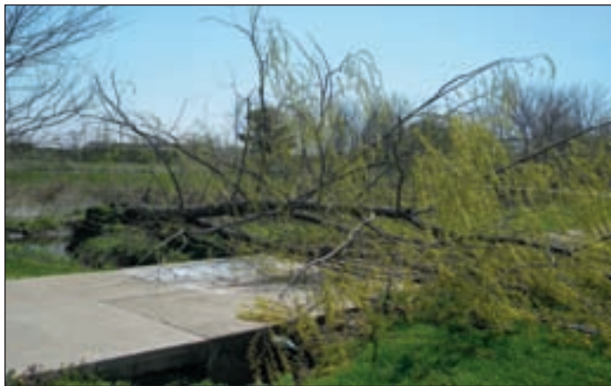
Research factors to consider regarding external forces: weather damage from wind, snow, and ice; site factors, such as saturated soils and slope; and rapid changes in dynamic loading.
