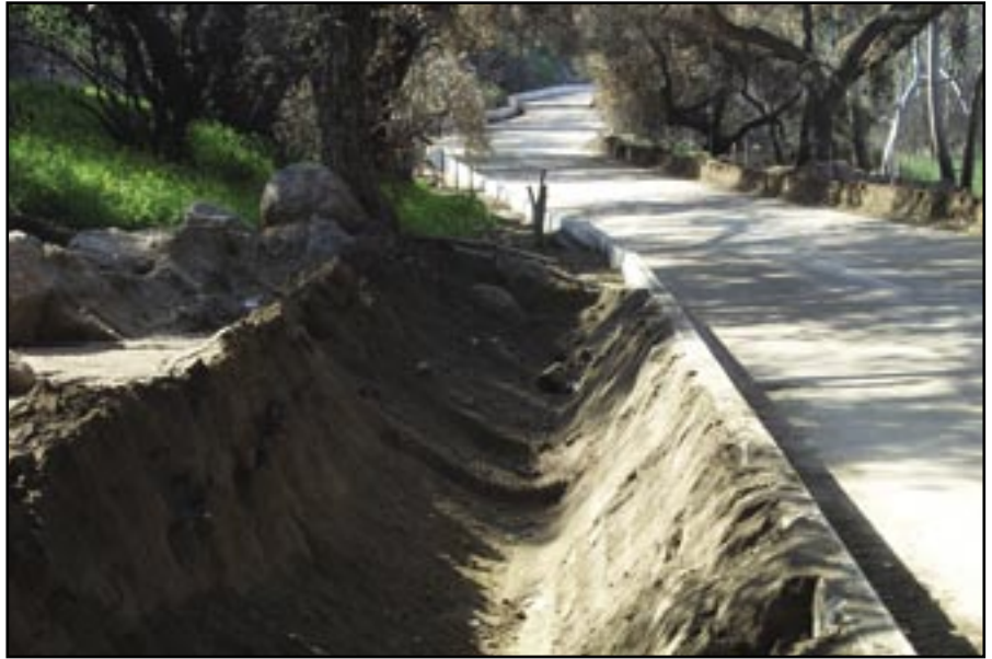
Figure 103—Jersey barriers (k-rails) line this road to protect vehicles on the road from debris flows.
