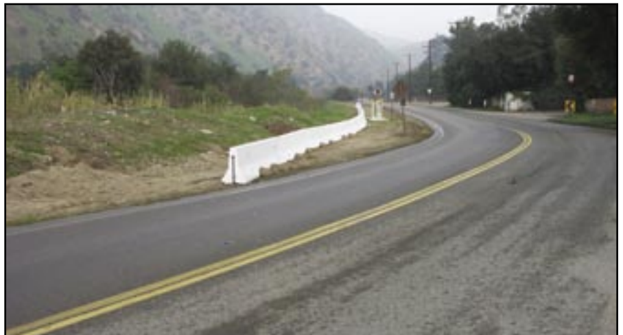
Figure 108—Jersey barriers can be removed from the road prism once the emergency is over.
