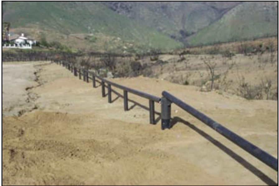
Figure 101b—Metal fencing to restrict vehicle access to an area that is naturally recovering.
