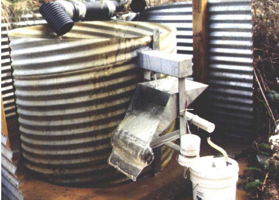
Figure 13. Tipping bucket and flow splitter in operation. The 20 gpm (66 lpm) design is shown.
